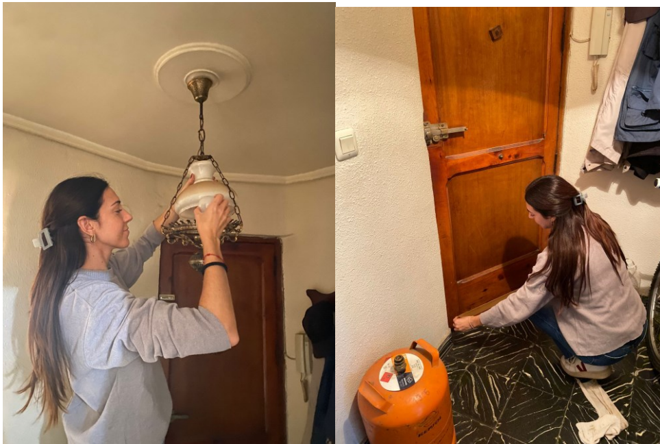
Figure 15 - Domestic intervention. Installing LED light bulbs and strip placed under the door to prevent cold air from entering or heat from escaping
